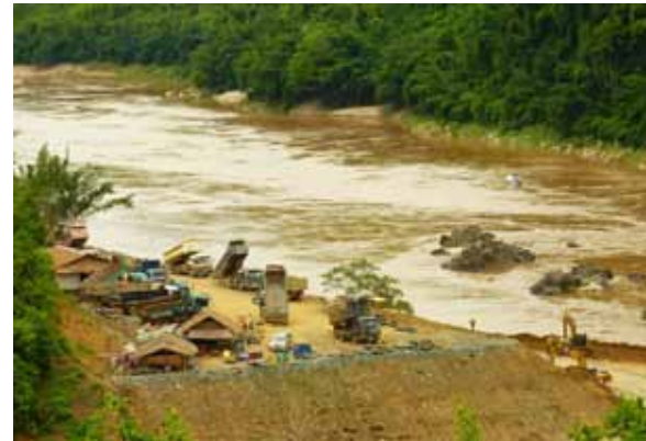
Construction of the Xayaburi dam in Laos. The Finnish firm behind Xayaburi's impact assessment report is facing an ethics complaint for alleged conflict of interest. http://www.flickr.com/photos/internationalrivers/7609214386/
